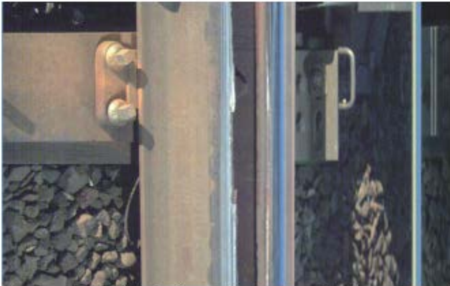
Material flaking in a switch
